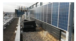
Green roof and PV panels
